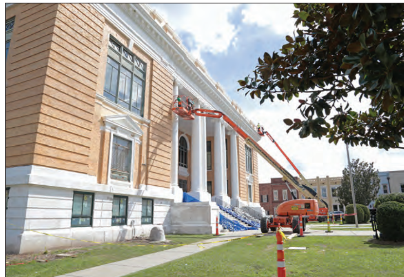
Sumter County Courthouse is renovated in October 2018 as part of a Penny for Progress project.
