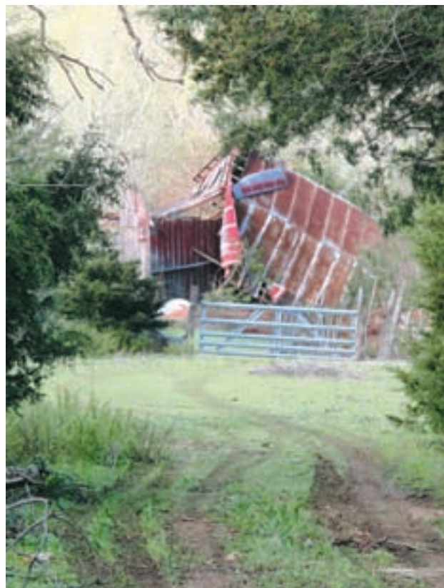
A barn near Kermit Road on Happy Hollow Road was heavily damaged by the storm. - Photos by Ed Schuh
