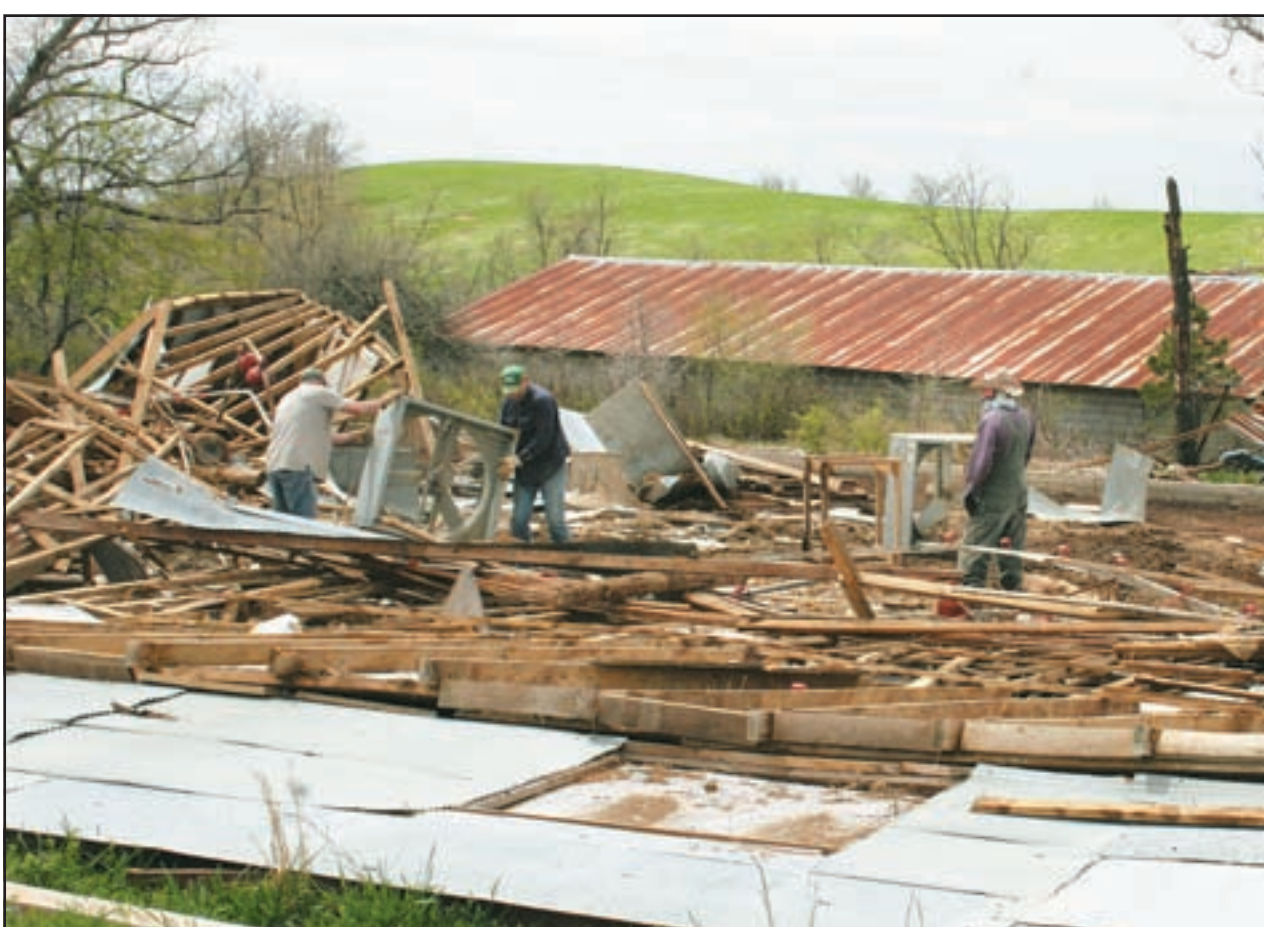
Rowdy and Steve Ross help their father, Tony, in clearing out equipment from the rubble of a former broiler house that was being used as a hay
