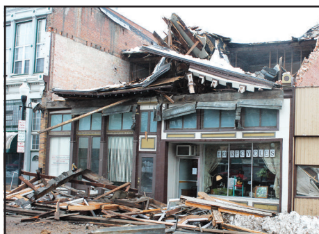
Feb. 22: The buildings at 118 and 114 - 116 N. Church St. collapsed. A loud roar and plenty of dust occurred when the building collapsed. No one was injured.
