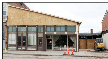
March 13: Much progress has been made after the collapse of the roofs on 114, 116 and 118 N. Church St. on Feb. 26. As this photo taken Monday afternoon shows, two weeks after the collapse, cleanup of the buildings is all but complete. Fayette City Inspector Angie Malone praised the owners of the collapsed buildings, Dan Reuther and Don Belcher, for promptness and thoroughness in repairing their buildings.
