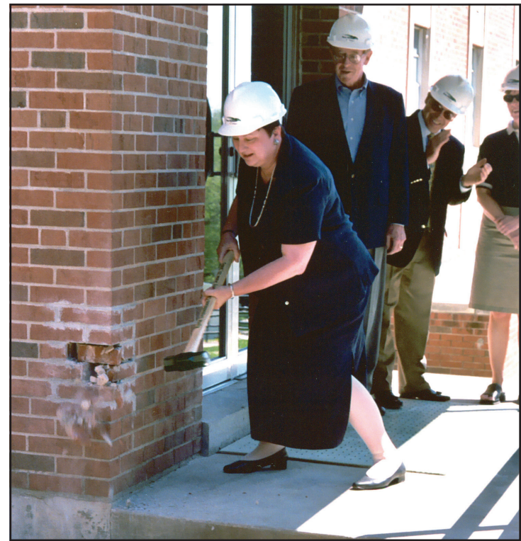
Dr. Marianne Inman swings the first sledge hammer to raze the 56-year-old “temporary” Eyrie Student Union in 2003 to make way for construction of the new CMU Student and Community Center which opened in 2005.
