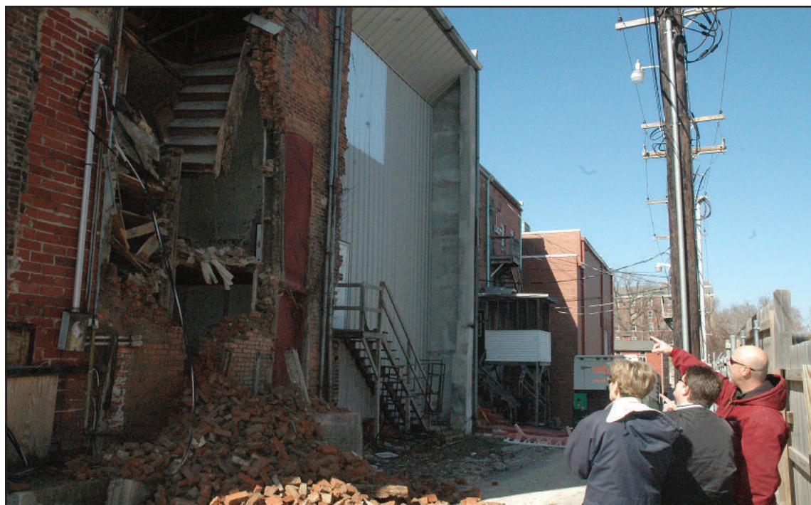
Stairs and floor joists are visible after the east wall of the former Colonial Mercantile building collapsed sometime Sunday night. Inspecting the wreckage on Monday morning are Mayor Jan Addison, Building Inspector Angie Malone and MECO engineer Jim Bensman.
